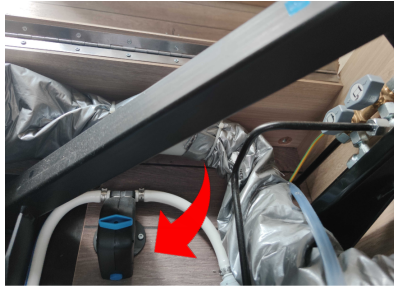
Fig. 6.2 –Anti-Frost drain valve location, positioned backwards behind black bar
